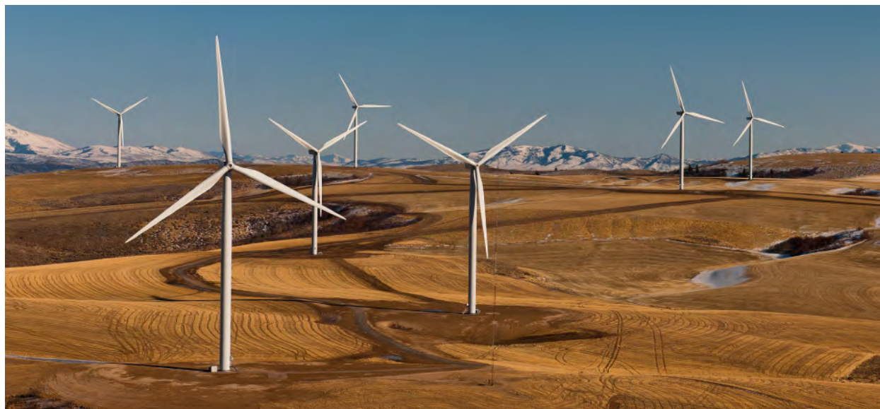
Figure 10.1 Brazos wind farm in west Texas. As of 2012, wind farms in the US had a power output of 60 gigawatts, enough capacity to power 15 million homes for a year. (credit: modification of work by “ENERGY.GOV”/Flickr)
